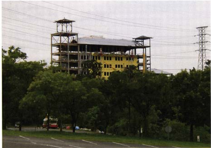
The $54 million structure at Montclair State University will feature a Spanish-mission style exterior envelope of cast stone and stucco, along with a clay tile roof. Construction began last year and wraps up later this year.
