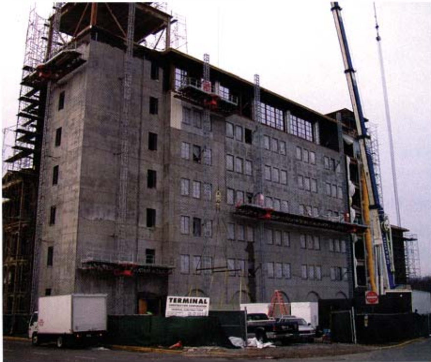
New Jersey's fastest-growing public university is adding a 266,000-sq.-ft. academic facility, the latest in a busy construction program on campus. The structural steel building will house the university's teacher education programs.
